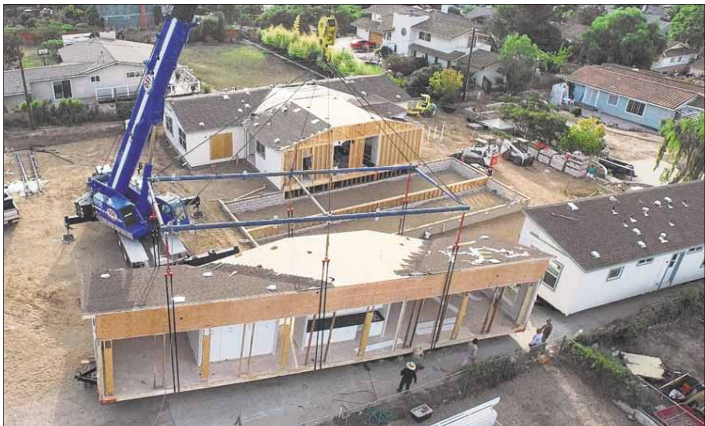
A crane lifts a portion of the home into place on the foundation.
